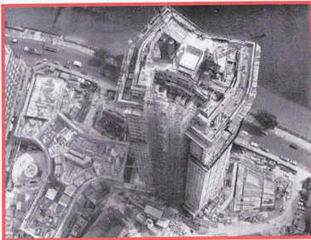
1962 Millbank Tower, London (Air conditioning by Ellis Mechanical)
