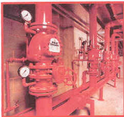
1970s Fire protection (How Group)
