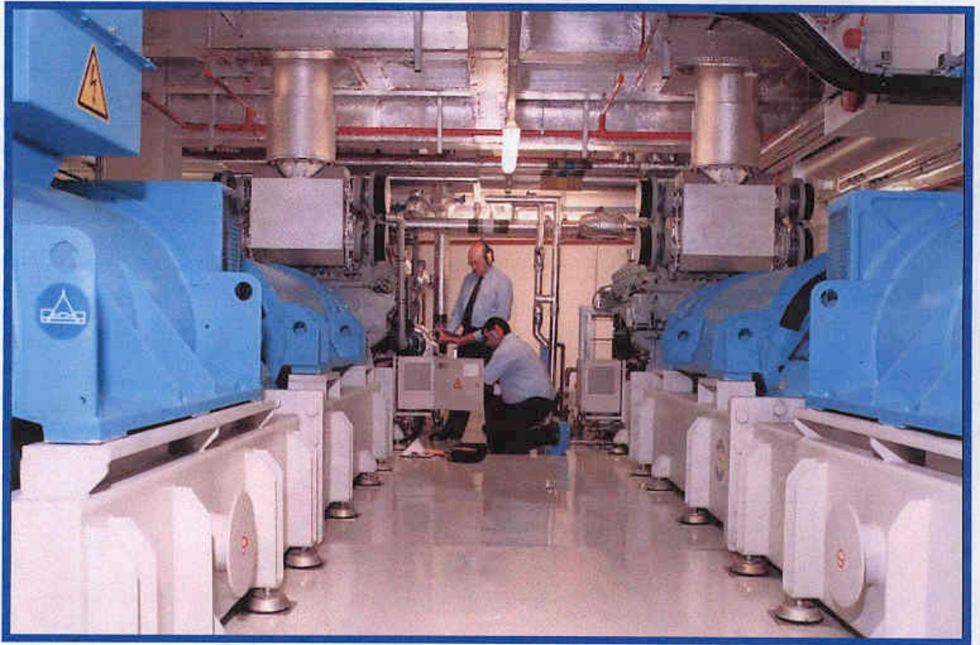
2003 Royal Bank of Scotland, Bishopsgate, London (UPS plantroom, operated and maintained by Lorne Stewart Plc)
