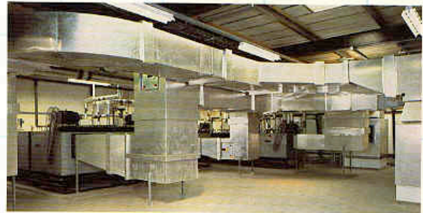
Seven of the plant rooms at the New Grimsby District Hospital have been supplied with Matthews & Yates air handling units and centrifugal fans.
