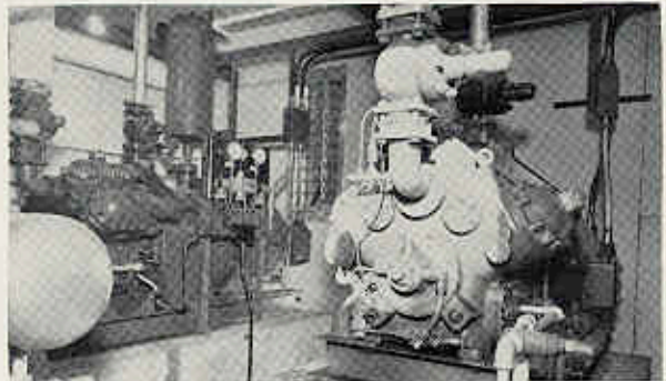
AIR CONDITIONING PLANT ROOM, ROWNTREE AND COMPANY LTD., YORK.
