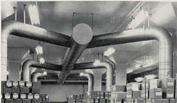
CLOSE CONTROLLED TEMPERATURE ROOM, CADBURY BROS. LTD., MORETON.
