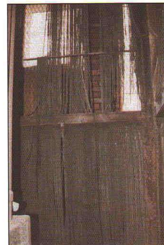
Coconut fibre rope filter wetted by sprinklers
