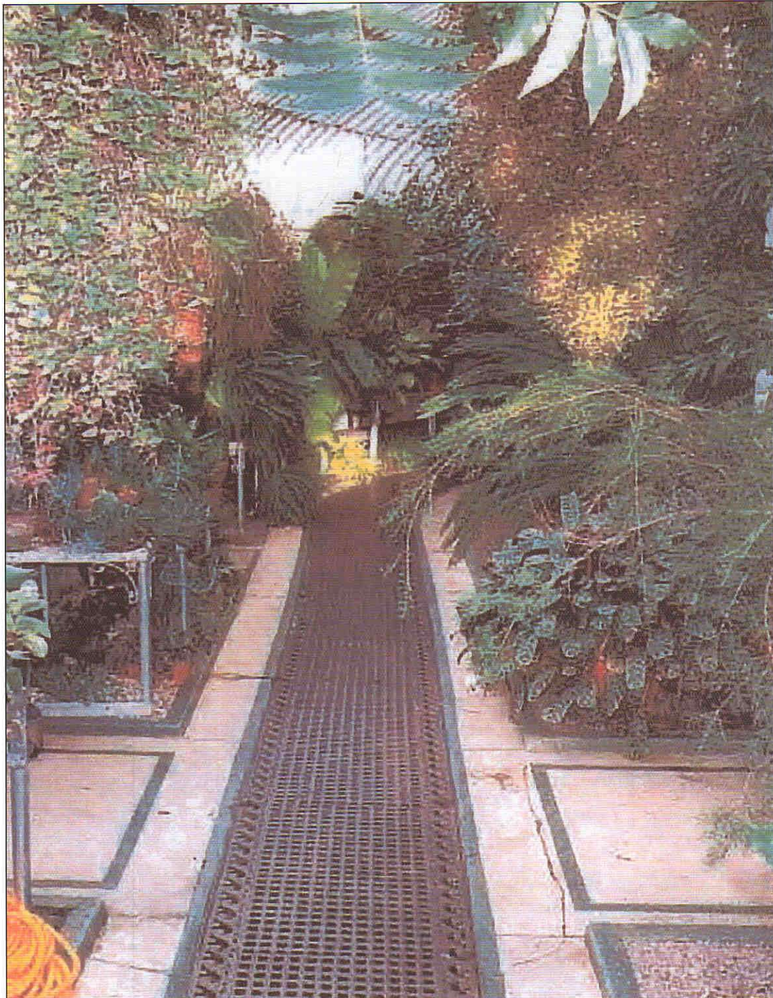
Heating duct with grating cover
