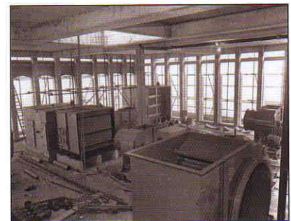
Air conditioning plant awaiting assembly 1962
