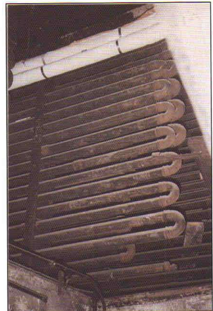
Existing heating coils
