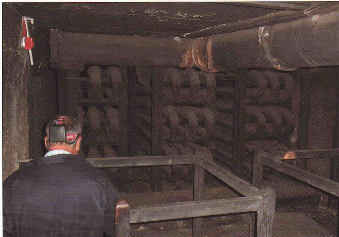
Heating chamber and coils as existing today
