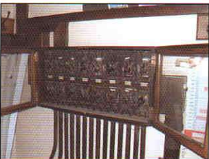
Electrical distribution board
