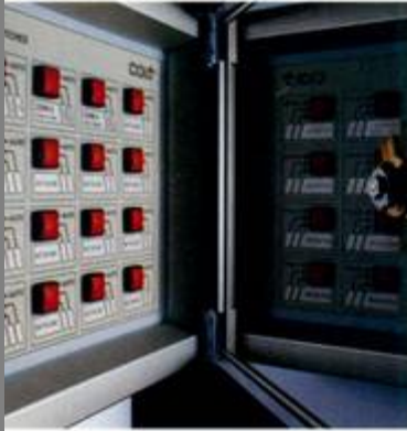
Right: The OPV control panel and the Fireman's override panel (above).
