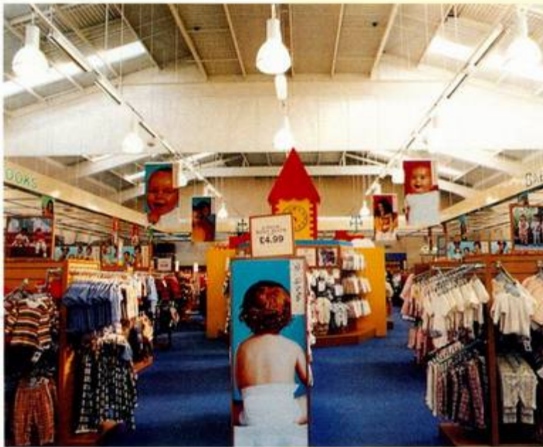
Children's World at West Quay Retail Park, Southampton is equipped with Colt Seefire natural louvred ventilators and a fixed smoke curtain. The smoke ventilation is controlled by the OPV system. The architects were BDP and Geoffrey Reid Associates.
