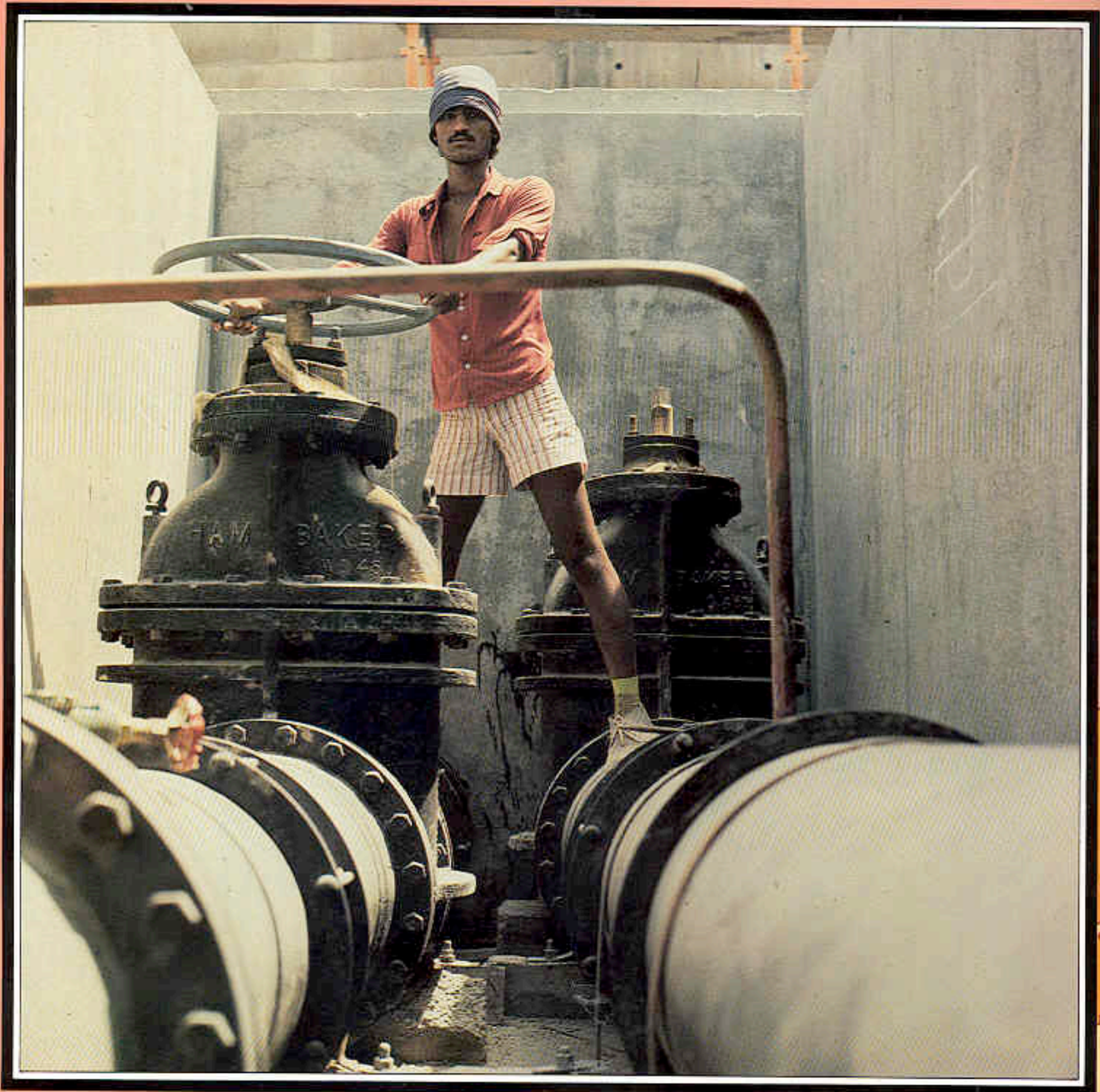
Above / Rashidiya Water Tank, Dubai, U.A.E. / Lunar Drake & Scull (U.A.E.) was responsible for all mechanical and electrical engineering services associated with the construction of this 12 million gallon water tank.
