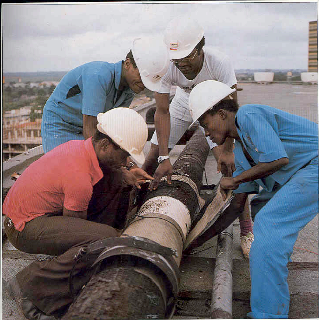
Above / Secretariat and Museum Complex, Port Harcourt, Nigeria / Drake & Scull (Nigeria) Ltd. was responsible for all electrical, mechanical, air conditioning, and plumbing services to this new complex.
