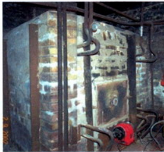
Perkins boiler in brick setting converted to oil-firing and still in use. Church of St Michael & All Angels, Bampton, Devon
