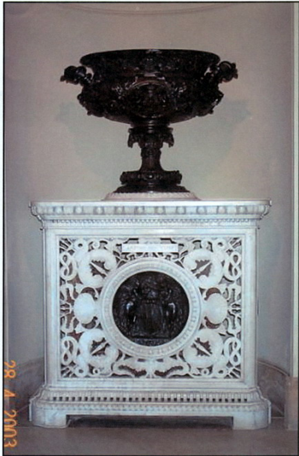
Italian marble radiator pedestal hiding double-bank pipe coil heater, Kingston Lacy, Dorset
