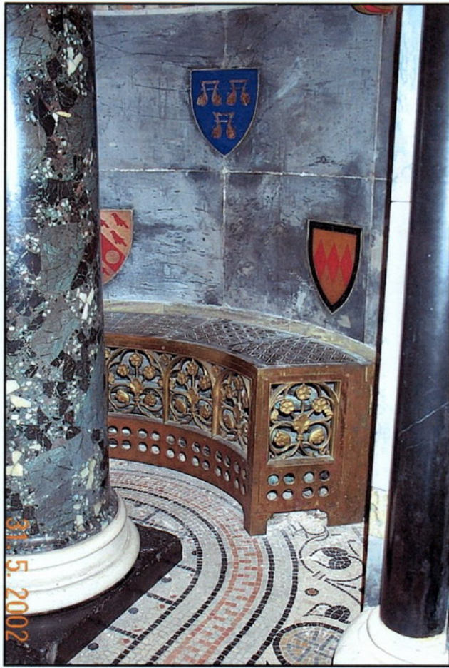
Decorative heating pedestal designed by William Burgess The heating engineer was Wilson Weatherley Phipson Cardiff Castle, c.1880
