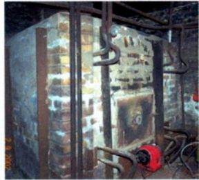
Perkins boiler in brick setting converted to oil-firing and still in use. Church of St Michael & All Angels, Bampton, Devon
