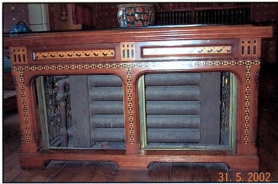
Box-end heating coil beneath Wm Burgess desk, Cardiff Castle. Heating designed by Wilson W Phipson, c.1880
