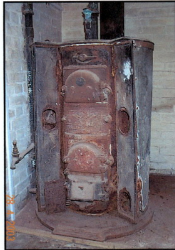
Lumby hot water service boiler, c.1900 discovered at Kingston Lacy
