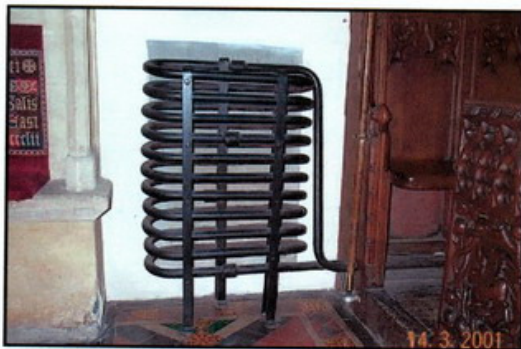
Perkins high-pressure hot water heating coil Church of St Mary, East Brent, Somerset
