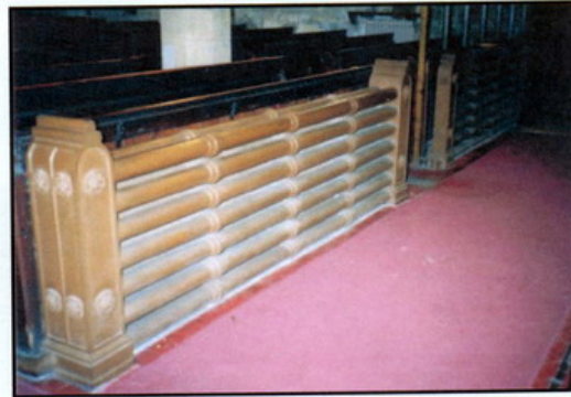
Box end heating coil, Church of St Swithin, East Retford, Notts
