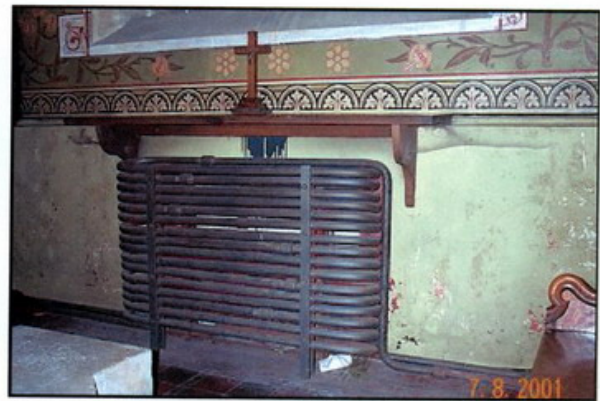
Perkins high-pressure hot water heating coil Church of St Thomas à Becket, Northaw, Herts
