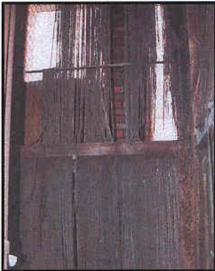
Air filter of coconut fibre ropes moistened by water sprinklers c.1900
