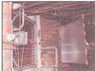
Branch duct to ward
