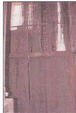
Coconut fibre rope filter wetted by sprinklers
