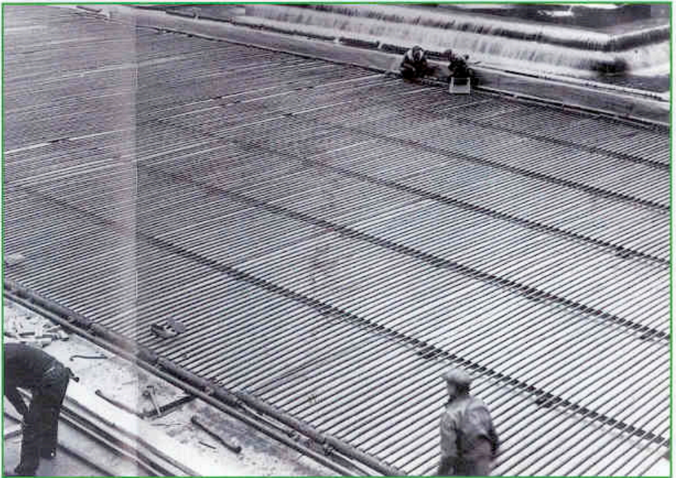
Ice skating rink. Laying the pipe grid. Rockefeller Centre, New York, 1936 [Works in Progress, pp.136-137]
