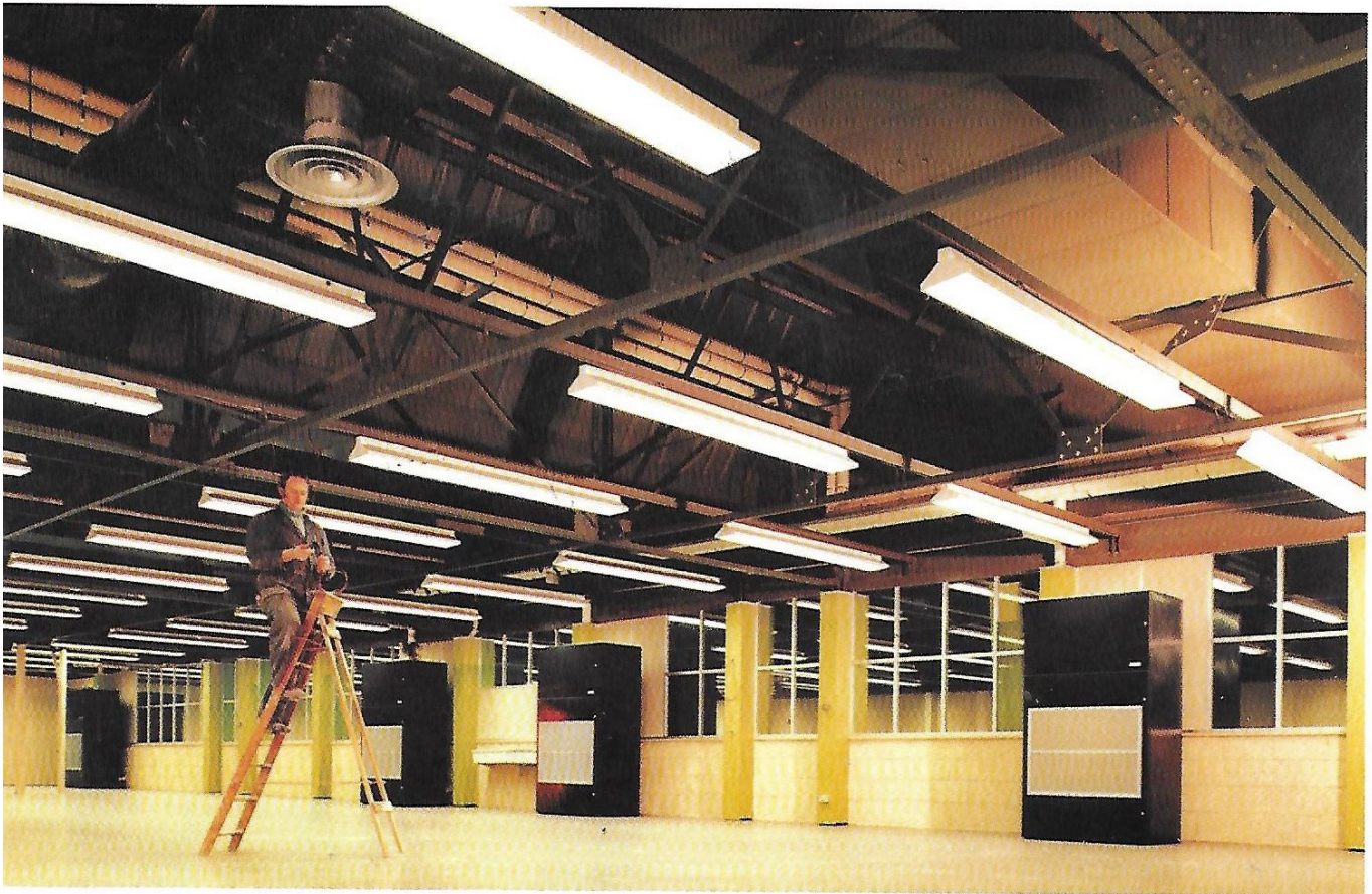
Above: Air handling units and overhead services in the Printing Works.
