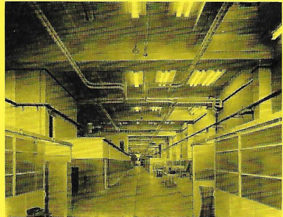
High Level Distributing Mains in BOAC Catering Headquarters at London Airport
