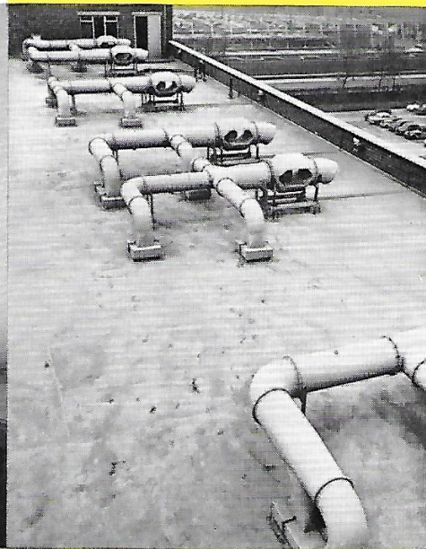
Fume cupboard extraction fans on roof of Research Building at The Imperial Chemical Industries Ltd, Billingham
