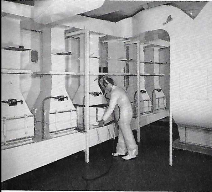
Changing contaminated filter cells at new laboratories for General Electric Co Ltd, Erith
