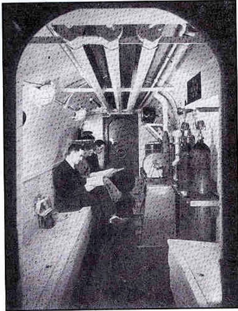
Demonstration Air Raid Shelter for 10 people, 1937, with CEC gas defence filtered ventilation system installed at 24 Buckingham Gate, London. [HVE, October 1937, 187].
