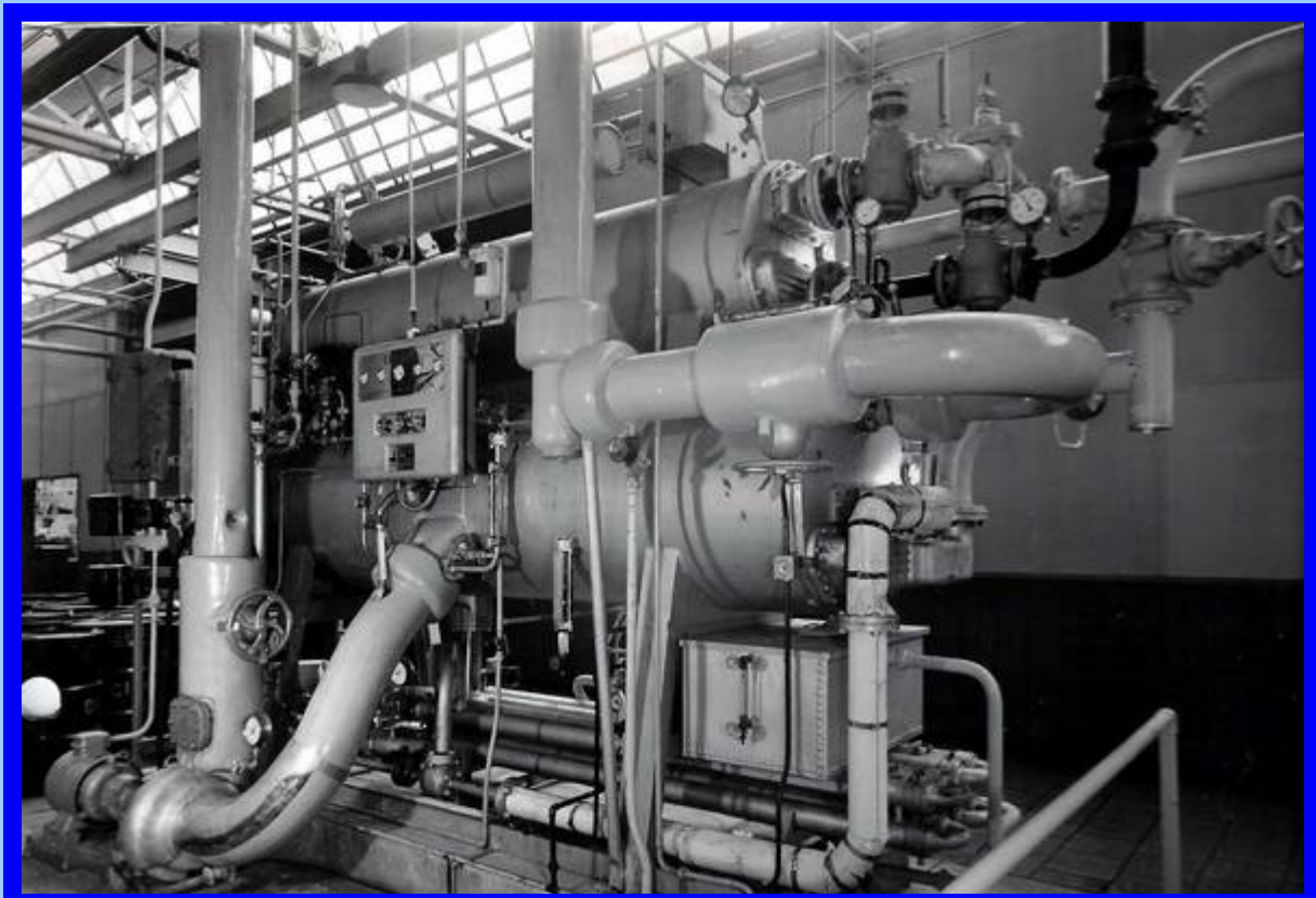
Carrier absorption machine of 150 TR (525 kW) installed at Mars Ltd, Slough c.1950
