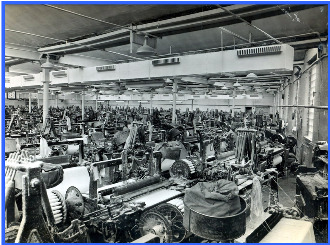
Carrier installation for a Weaving Shed at No. 2 Mill, Rock Nook for Sladon Wood, 1949 (CIBSE Heritage Group Collection)
