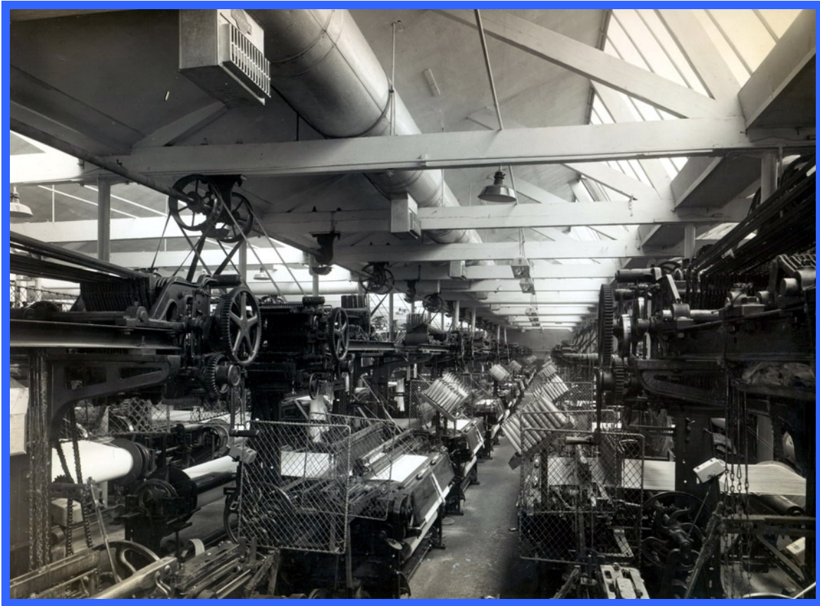
Carrier installation in a Weaving Shed for Gartside & Company, Waterside Mill, 1950 (CIBSE Heritage Group Collection)
