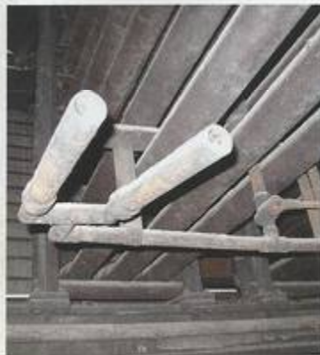
Figure 1: Steam injectors below main heating coil
