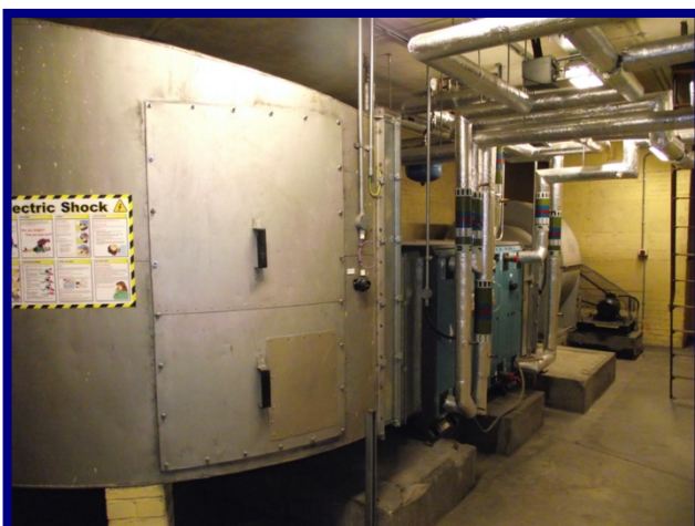
The Council Chamber air handling unit
