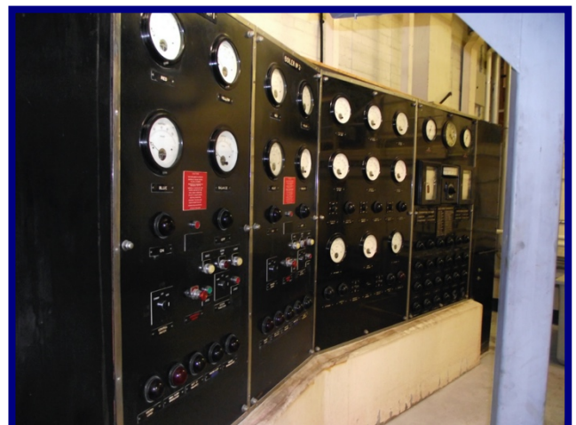
Boiler Room control panel
