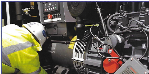
Standby Diesel Electric Generator Set
