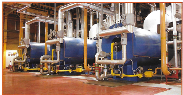
Gas-fired Steam Boilers at Bedford Hospital 2017
