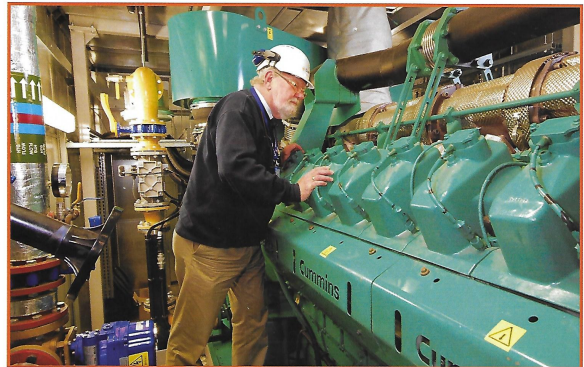
Southampton University Hospital doubles CHP (Combined Heat and Power) Capacity 2013
