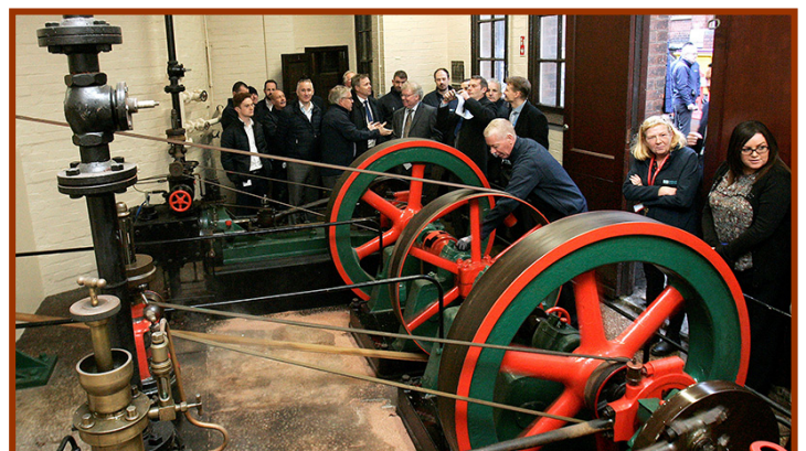
Steam Engines Royal Victoria Hospital, Belfast
