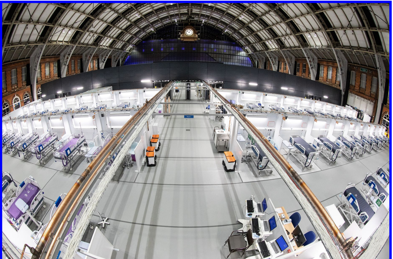
Arrangement of the Bed Stations each with oxygen and electricity
