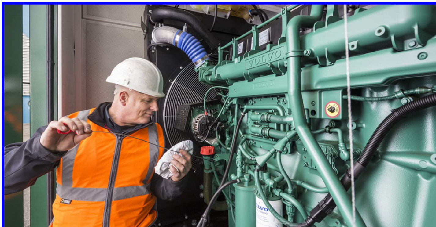
Checking standby diesel generator
