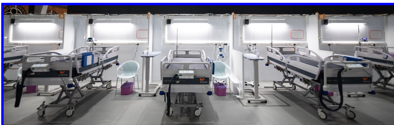
A view of completed bed stations each with oxygen and electricity
