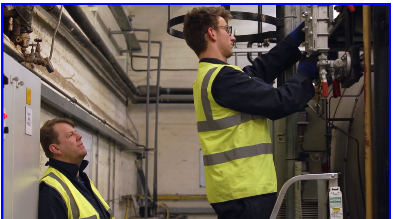
Maintaining piping, fuel lines and controls
