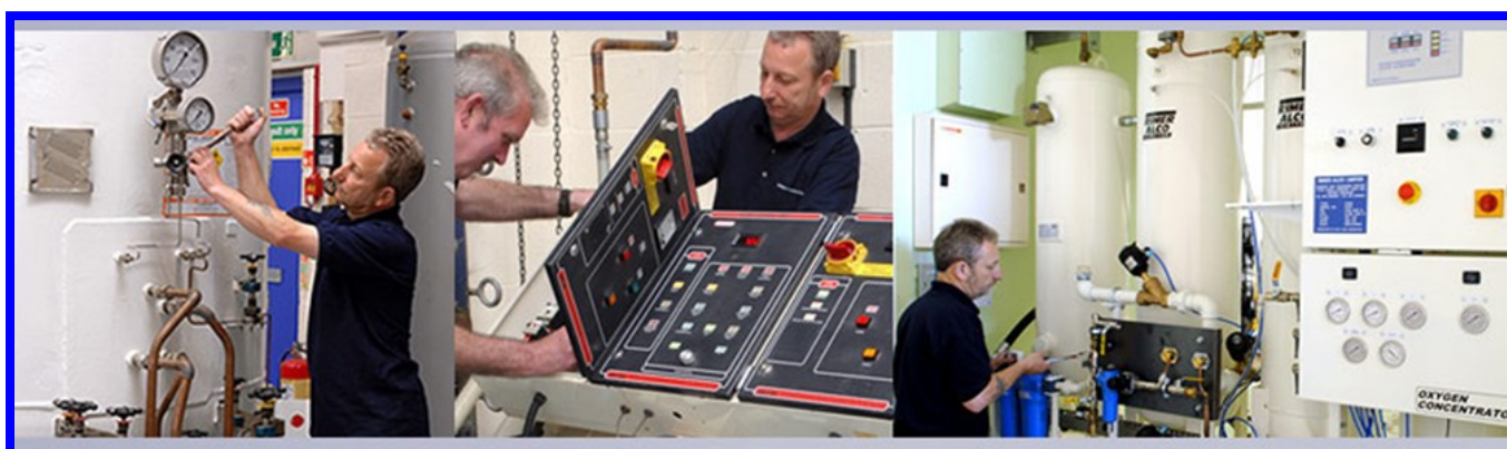
Medical Gases: systems and equipment
