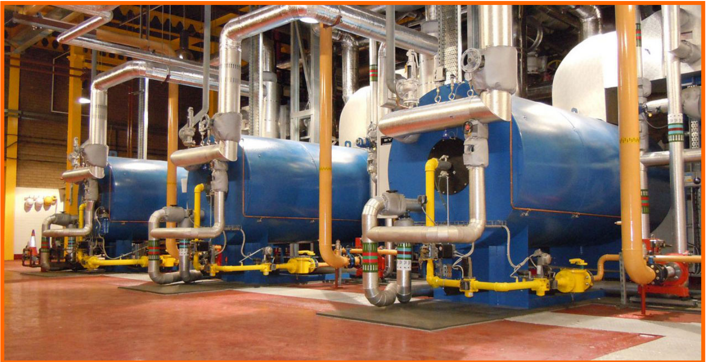
Gas-fired Steam Boilers at Bedford Hospital 2017
