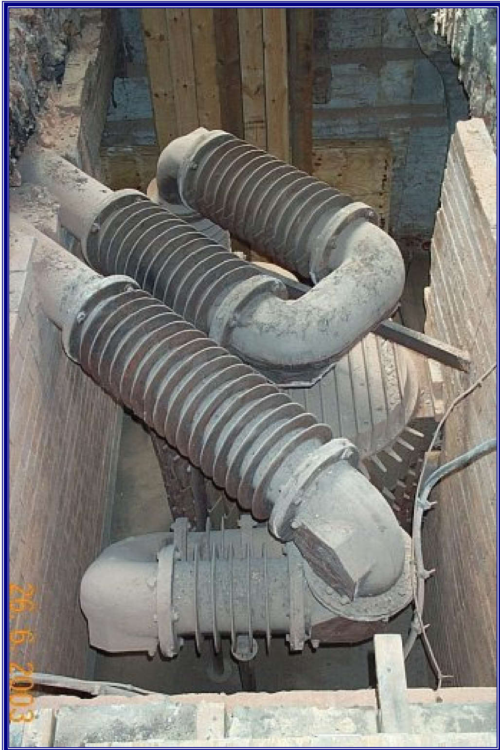
Grundy stove, St Paul's Church, Deptford, London
