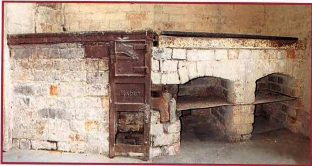
1830 G & J Haden installed a kitchen stove with a baking oven in Dinton House [FJF]
