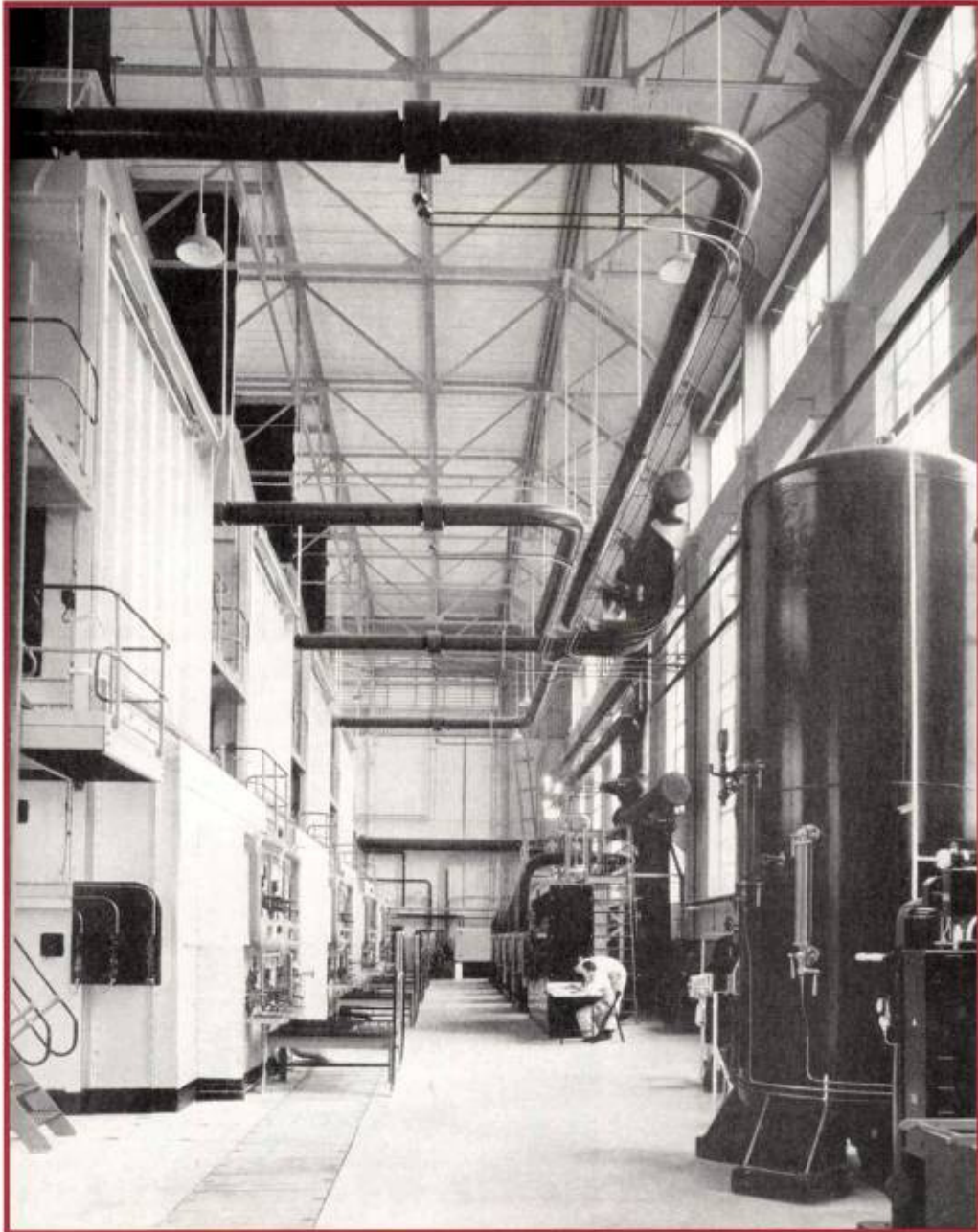
Leyland Motors Ltd, Ministry of Supply Factory, Lancashire Heating by HPHW working at 225 psig provided by four boilers with a total capacity of 184 million Btu/h and with waste heat reclaim from diesel generators and the rubbish incinerator Architect Harry S Fairhurst & Sons
