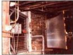
Branch duct to ward
