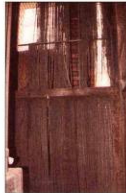
Coconut fibre rope filter wetted by sprinklers
