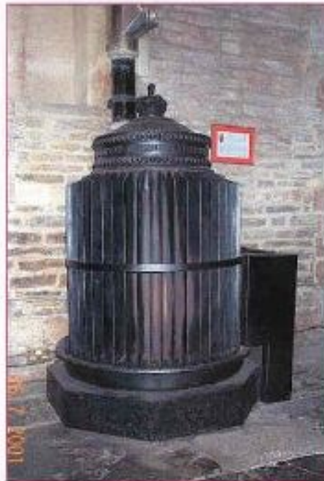
Gurney warm air stove at Tewkesbury [Heritage Group Collection]
